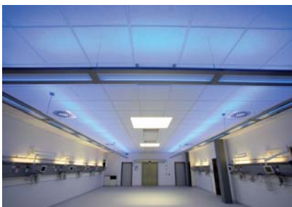
Figs. 2 to 4. The U-shaped array of BlueMotion luminaires from Trilux supplements the general lighting in the recovery room (photo: Trilux)
